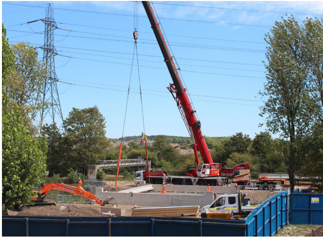
Construction works to open up the eastern side of the EcoPark, linking to the Laydown Area
