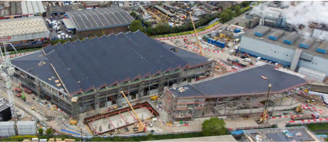
Aerial View of the EcoPark South project under construction, with the RRF in the foreground
