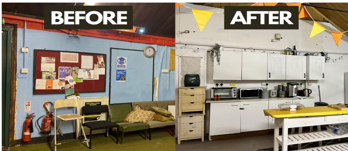
Progress made at St Barnabas Church in Waltham Forest, as a result of the Re-Power Communities Programme.
