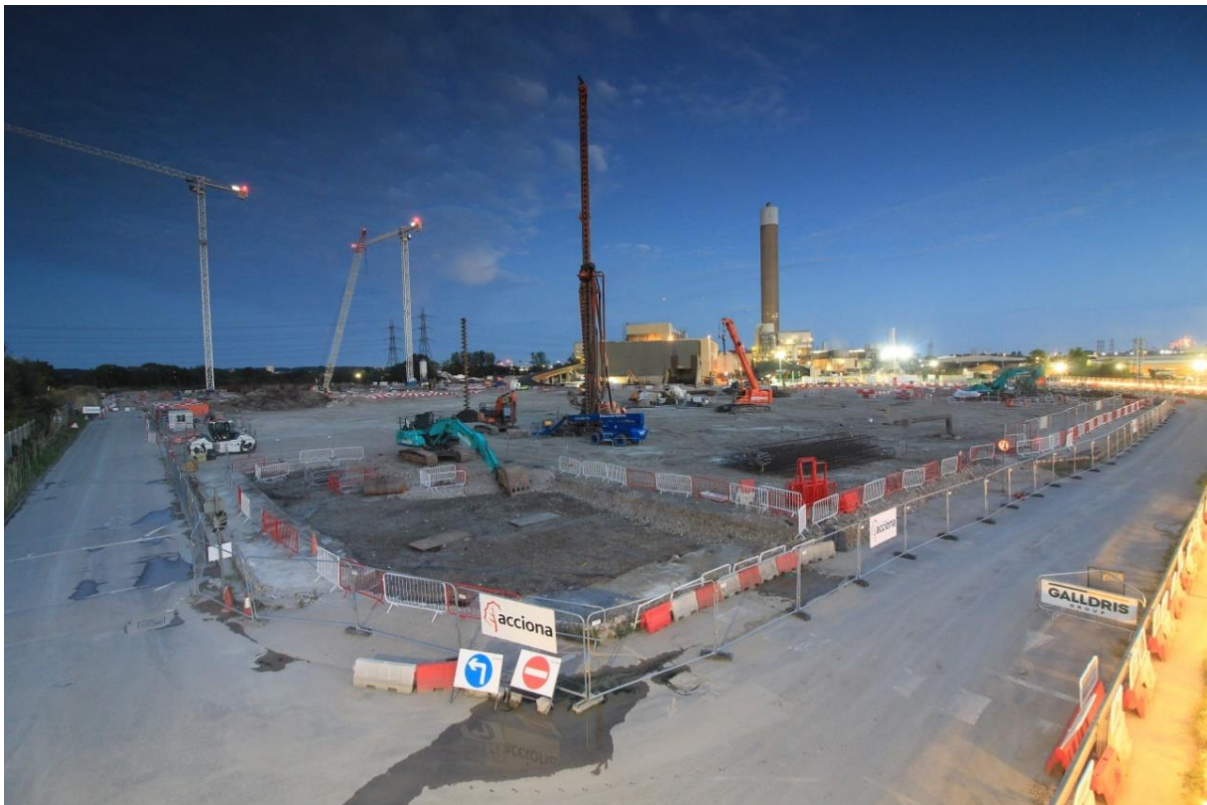
Phase 2 piling works in the western area of the site (two tower cranes in background)
