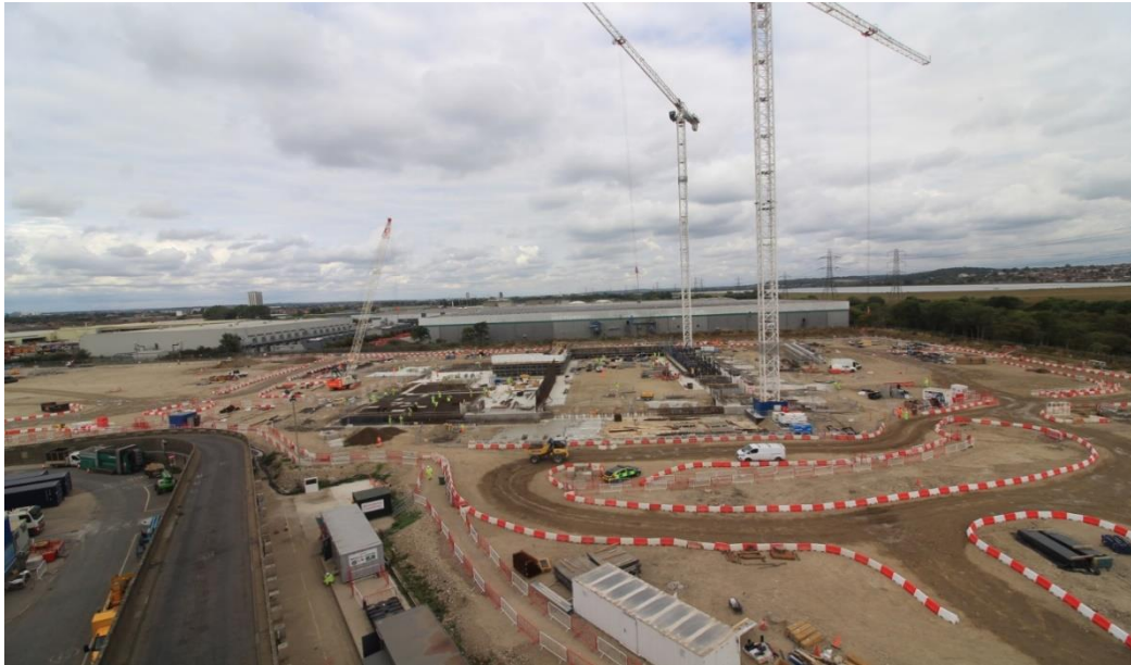
Figure 2: A view of the boiler and bunker areas and preparations for the slipform works
