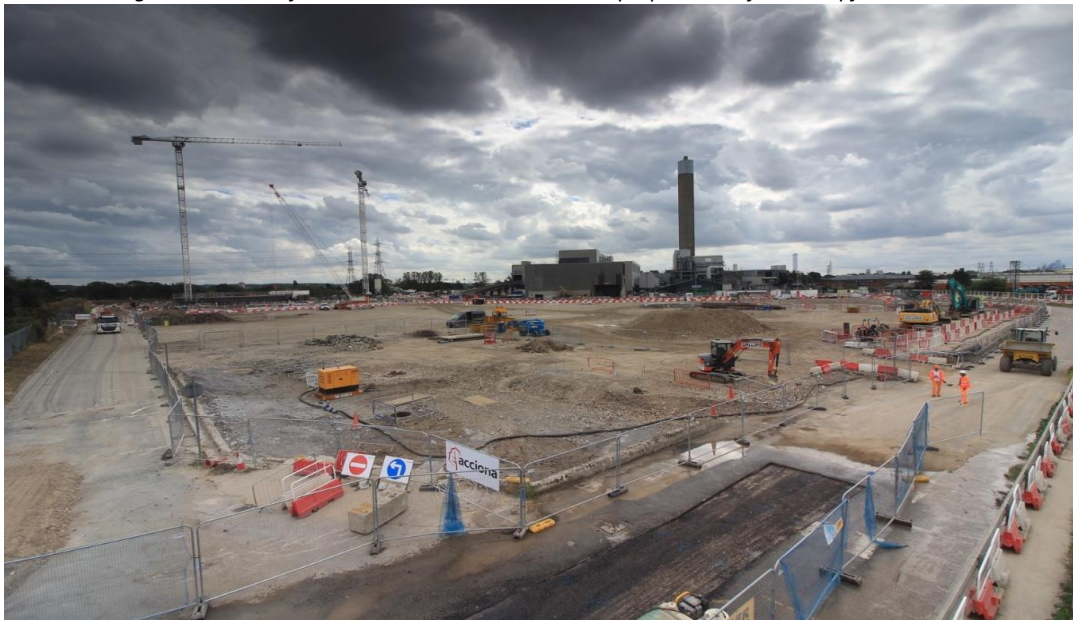
Figure 3: Completion of the second phase of piling and final enabling works (tank removal)
