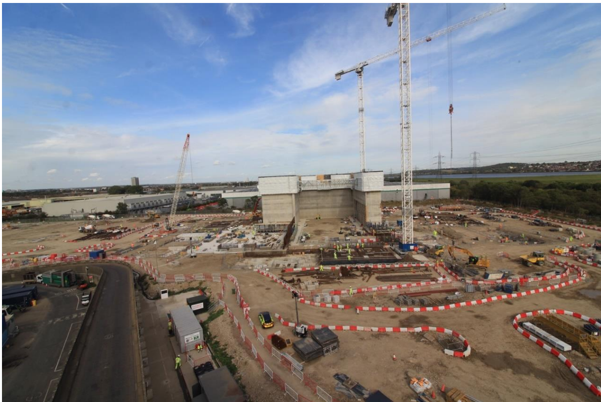
Figure 3: A view of the boiler and bunker areas and preparations for the slipform works.
