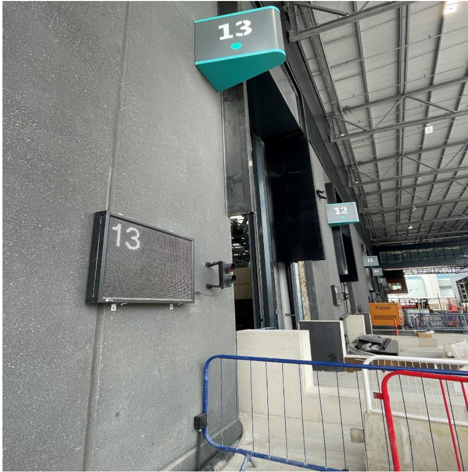
Figure 6: Waste bay display screens connected for testing
