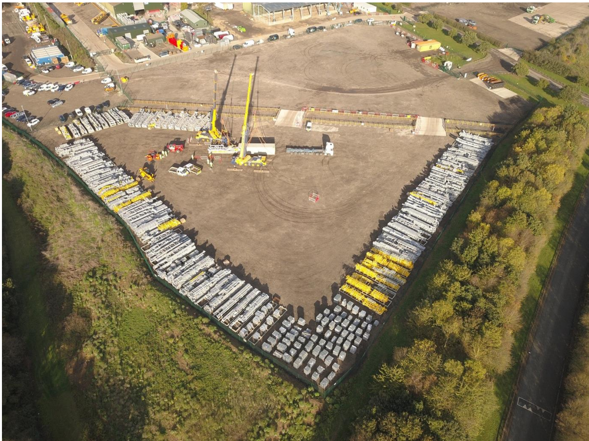
Figure 5: Deliveries of boiler and structure steel from HZI at Acciona's storage facility readiness for the commencement of boiler and structural steel erection
