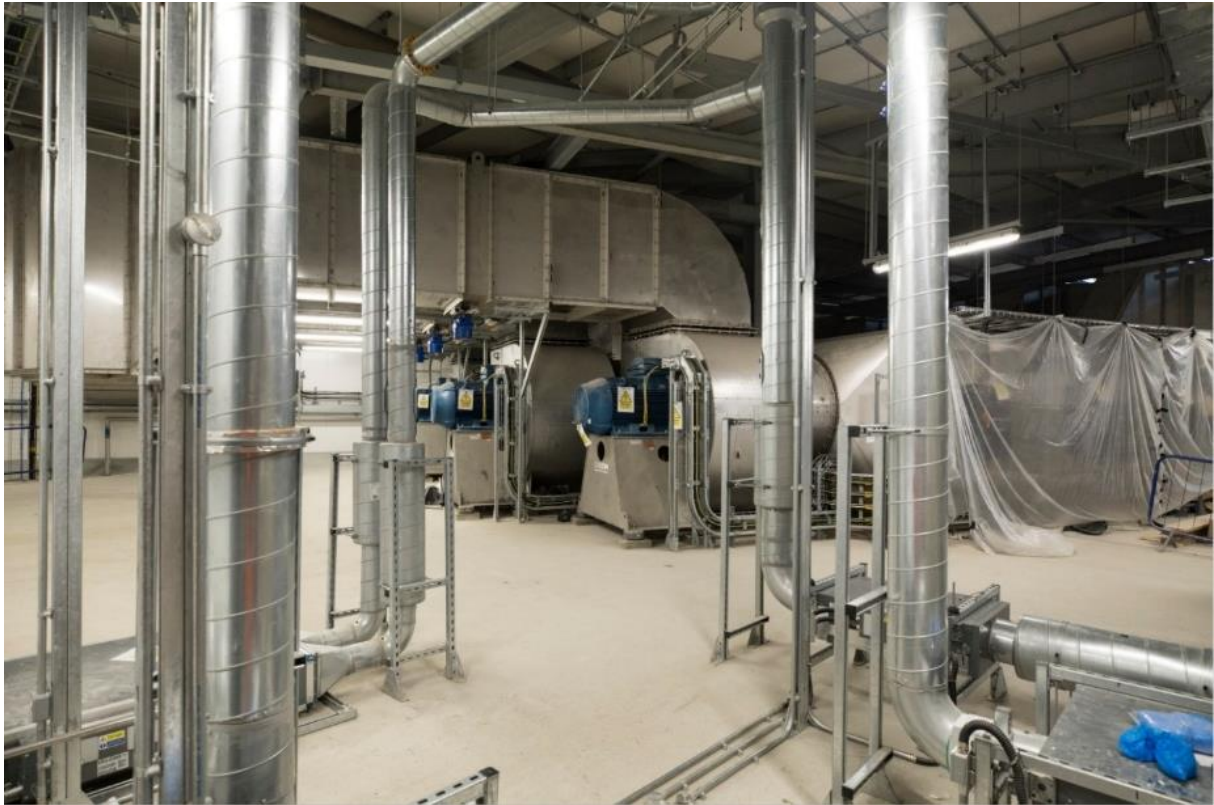
Figure 3: RFPF Integrated odour and Ventilation system ready for wet waste testing
