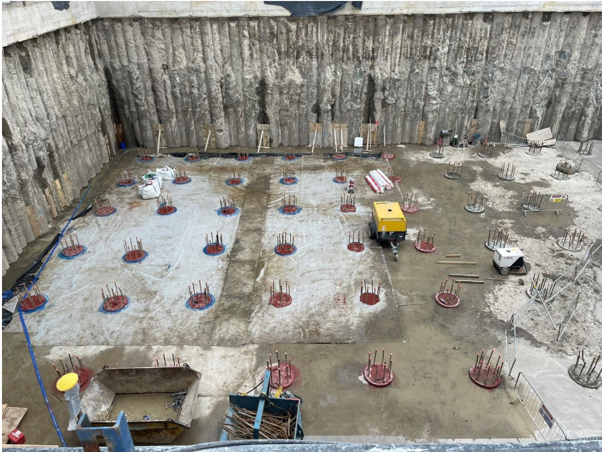
Figure 4: Completion of the bunker excavation and preparations for the installation of the mechanical tower crane
