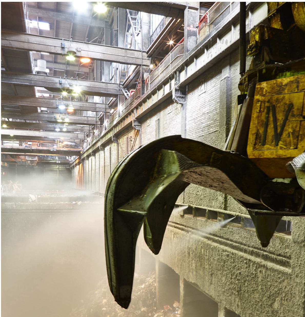
Waste bunkers at the EcoPark energy from waste facility
