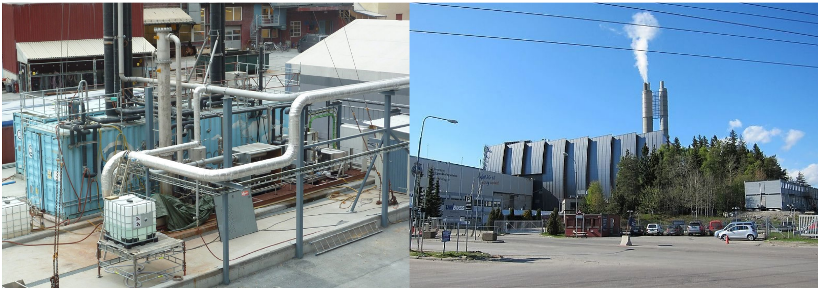
Figure 19: Klemetsrud EfW facility (right: Aker Solutions test plant at Klemetsrud, left: Klemetsrud EfW front view)
