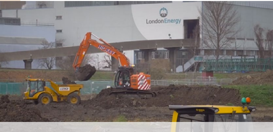
Image 1. Construction work on the Laydown Area, North London Heat and Power Project
